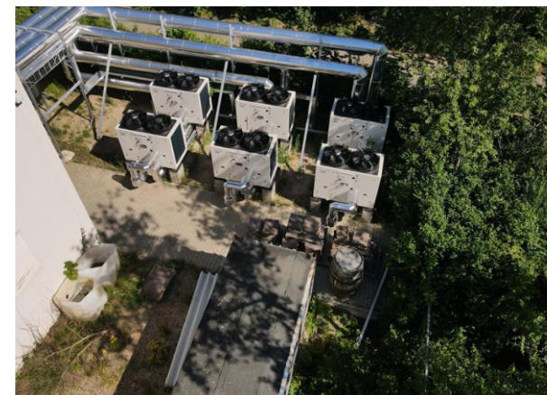
Heat pumps at the R&D site in Lüneburg, Lower Saxony, Germany
